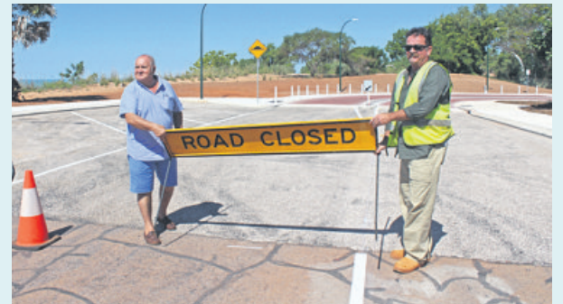
Shire President, Ron Johnston, and Shire Senior Project Engineer, Mark Renwick, open the connection of Dampier Tce and Frederick St. has also included the Jetty to Jetty Project, clean-up of Streeter's Jetty and installation of signage and interpretive information, undergrounding of power lines, additional shade trees and structures and expanding Christmas lighting and decorations," Mr Donohoe says.
