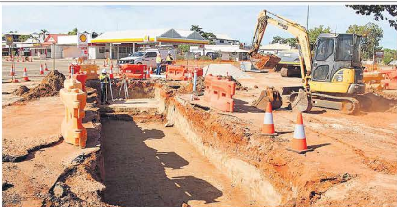
The intersection of Hamersley St and Napier Tce is undergoing upgrades for safety and drainage.
