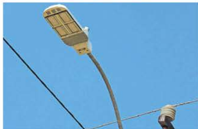
Community members are encouraged to report faulty street lights to Horizon Power.
