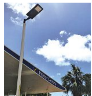
The Shire has rolled out 18 solar lights in the Broome Visitor Centre carpark.
