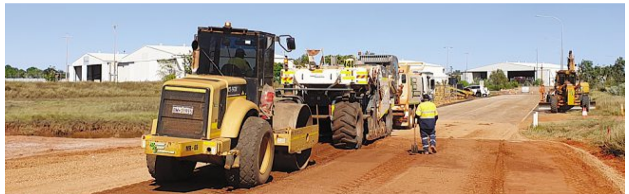
Works are progressing on the Gus Winckel Intersection Upgrade, with major earthworks taking place last week.
